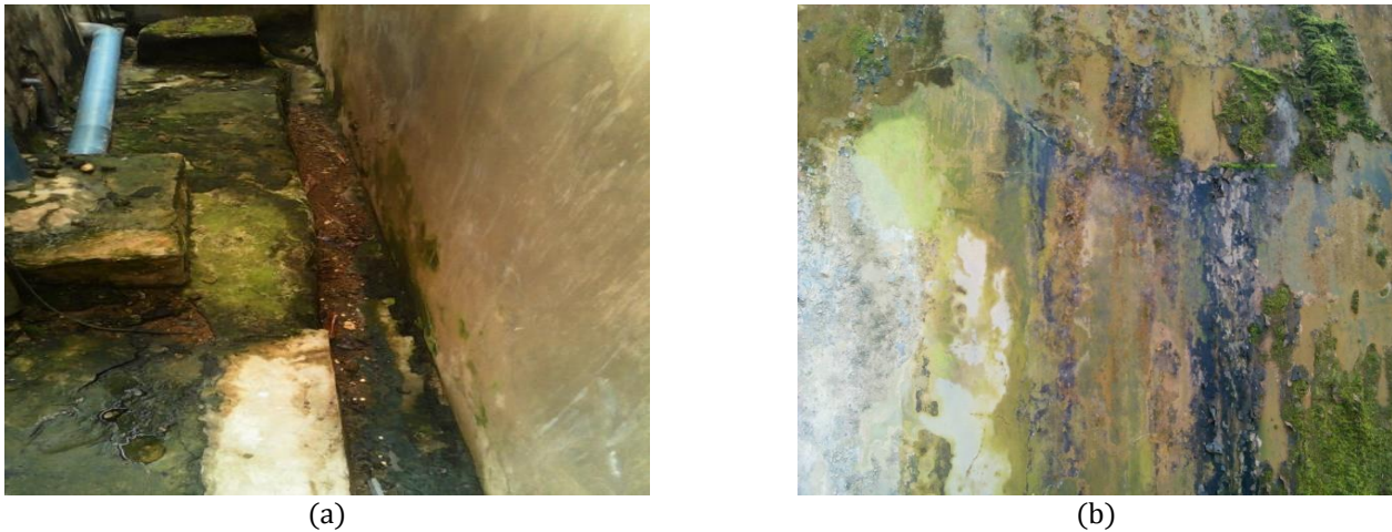
Figure 4: Typical concrete and steel corrosion (a) growth of algae (b) algae growing into the concrete
